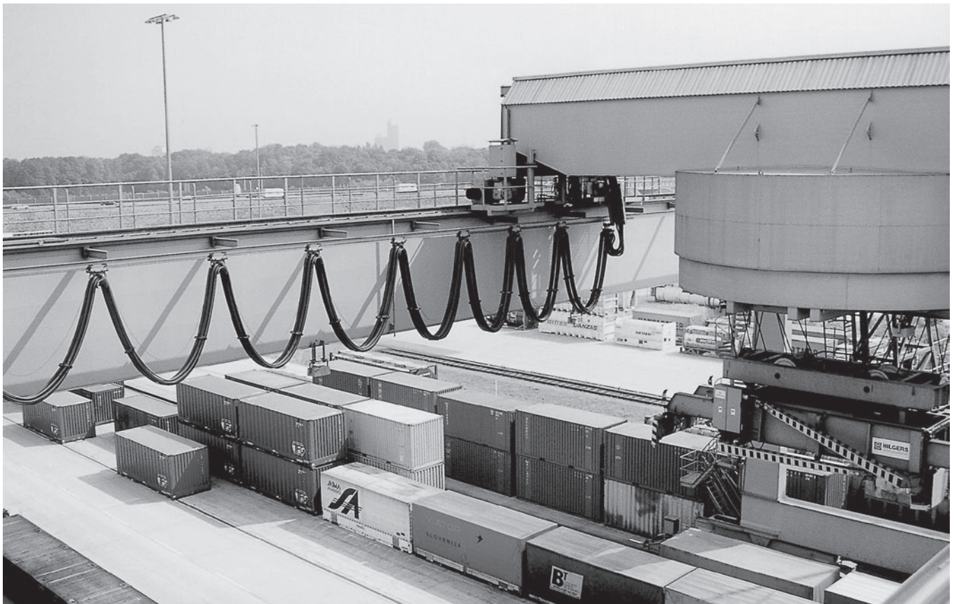
Cable carrier at a container crane
